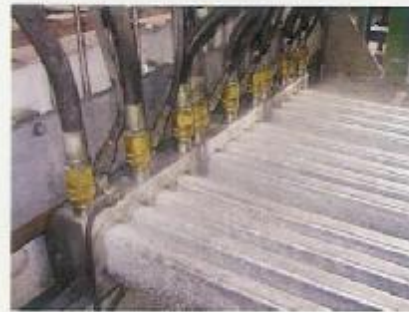
Fig. 2: View on ingot moulds and strands (note that water and lubricant connections are accessible from the top)
